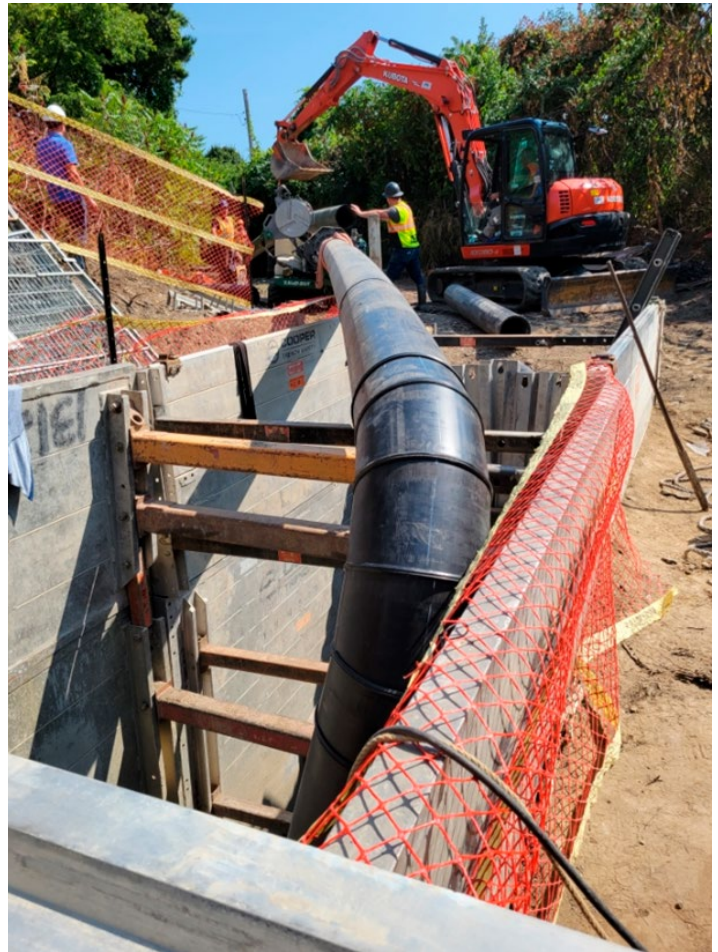
Connection of the overland HDPE by-pass pipe at the south side of the Queensway in progress.
