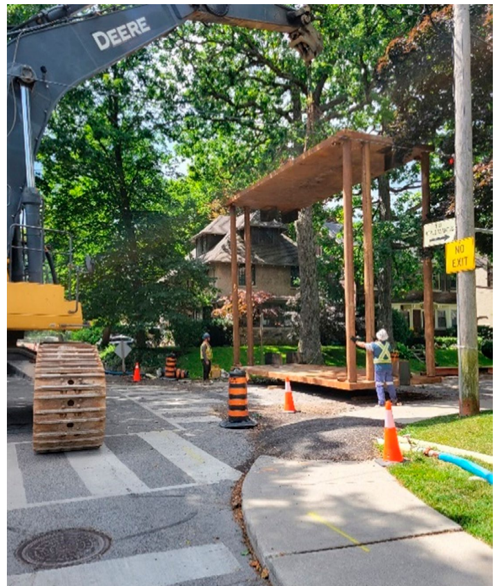
Transportation of the steel shoring box assembly to be installed at Ridge Drive excavation pit.
