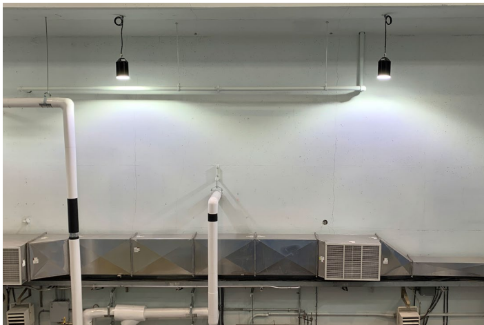
LED lights in the pump gallery, mounted approximately 14.5 m above the basement floor.
