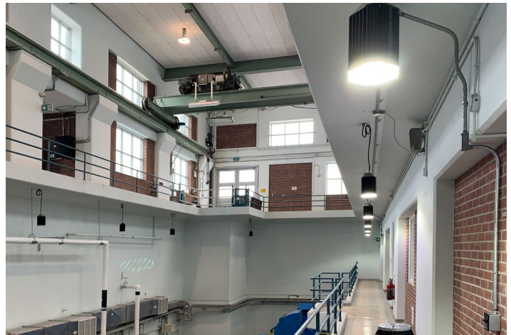
A wide view of the high-bay LED lighting fixtures in the pump gallery, part of the award-winning lighting project at Parkdale Pumping Station.
